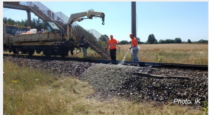
Photo. 2 Resin application on an illegal crossing on the Test Track in Żmigród
