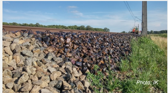
Photo. 1 The end of the superstructure section covered with resin on the curve R = 900 \text{ m}
