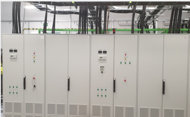
Fig. 1. The view of the multi-system substation traction converter
