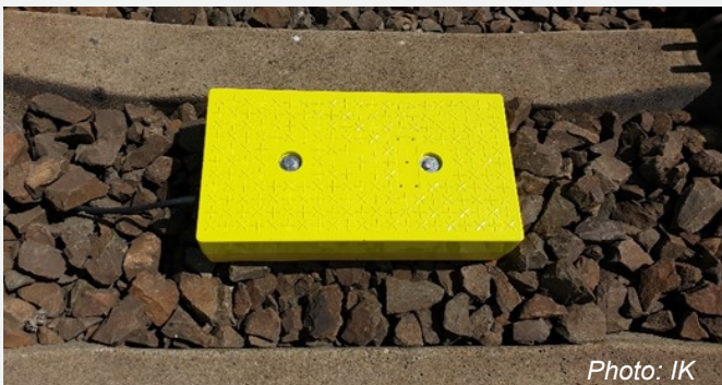
Fig. 1. Eurobalise prototype on the Test Track Centre
