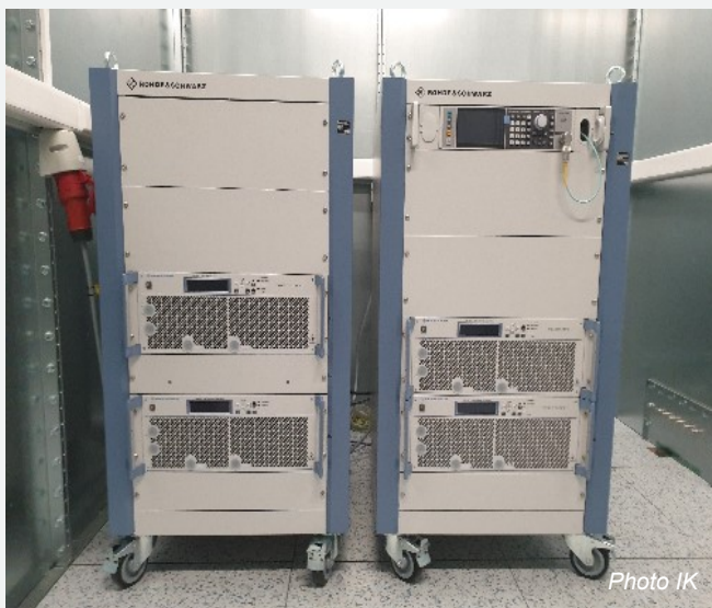
Photo 1. View of installed EMS measuring system equipment in a rack system
